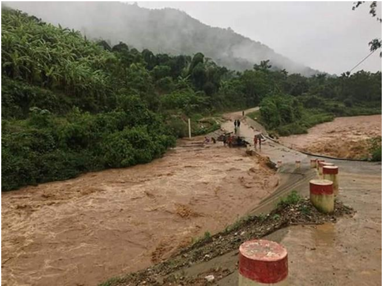
A road is damaged after heavy rain in Muong Lat district, Thanh Hoa province (Photo: VNA)
